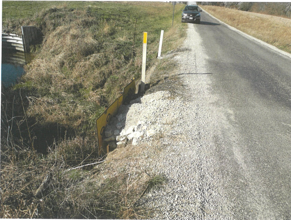
Rural – 1800N 900E 10' x 5' needs 40 feet 96" to Flowline Severe cracking, box floor gone, road undermined
