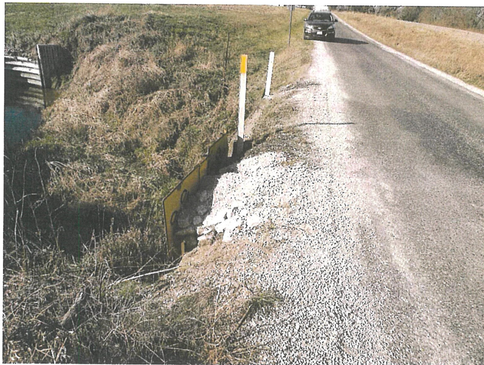
Rural – 1800N 900E 10' x 5' needs 40 feet 96" to Flowline Severe cracking, box floor gone, road undermined
