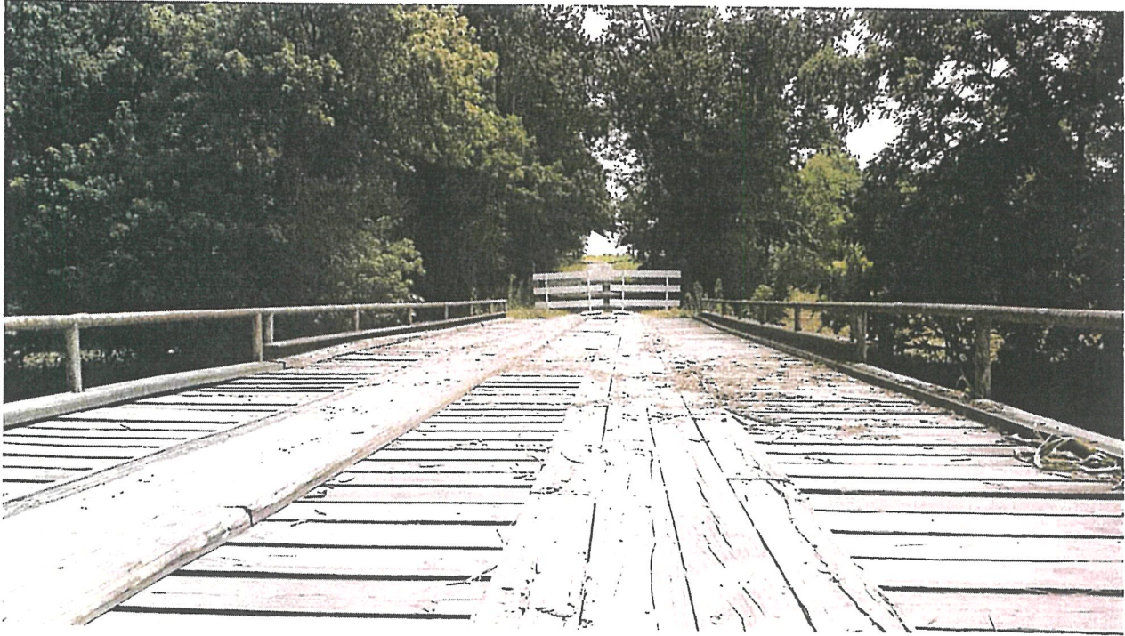
Standing at West Abutment, facing East. Debris has been removed from under deck boards.
