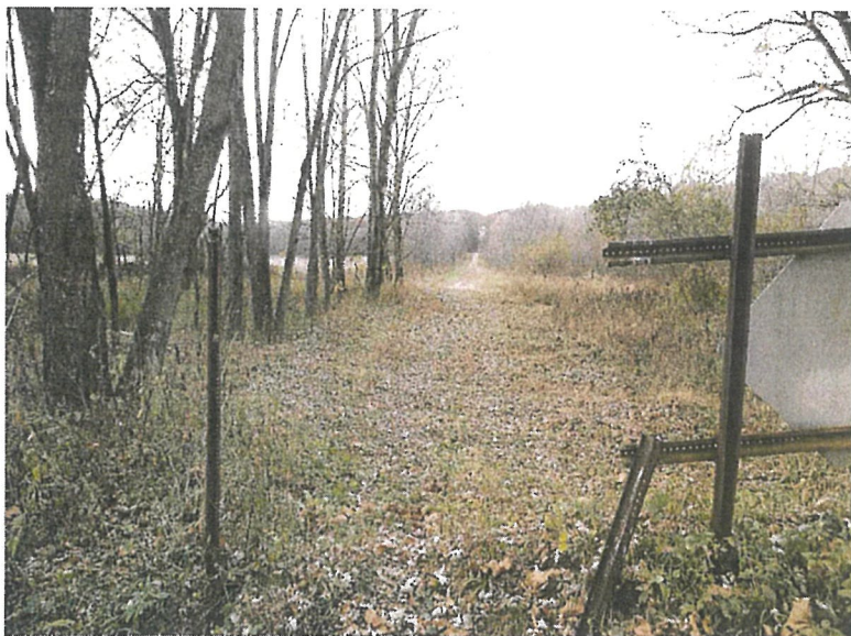
Herrick bridge 087-3062 – Closed to Traffic; 130 feet long
