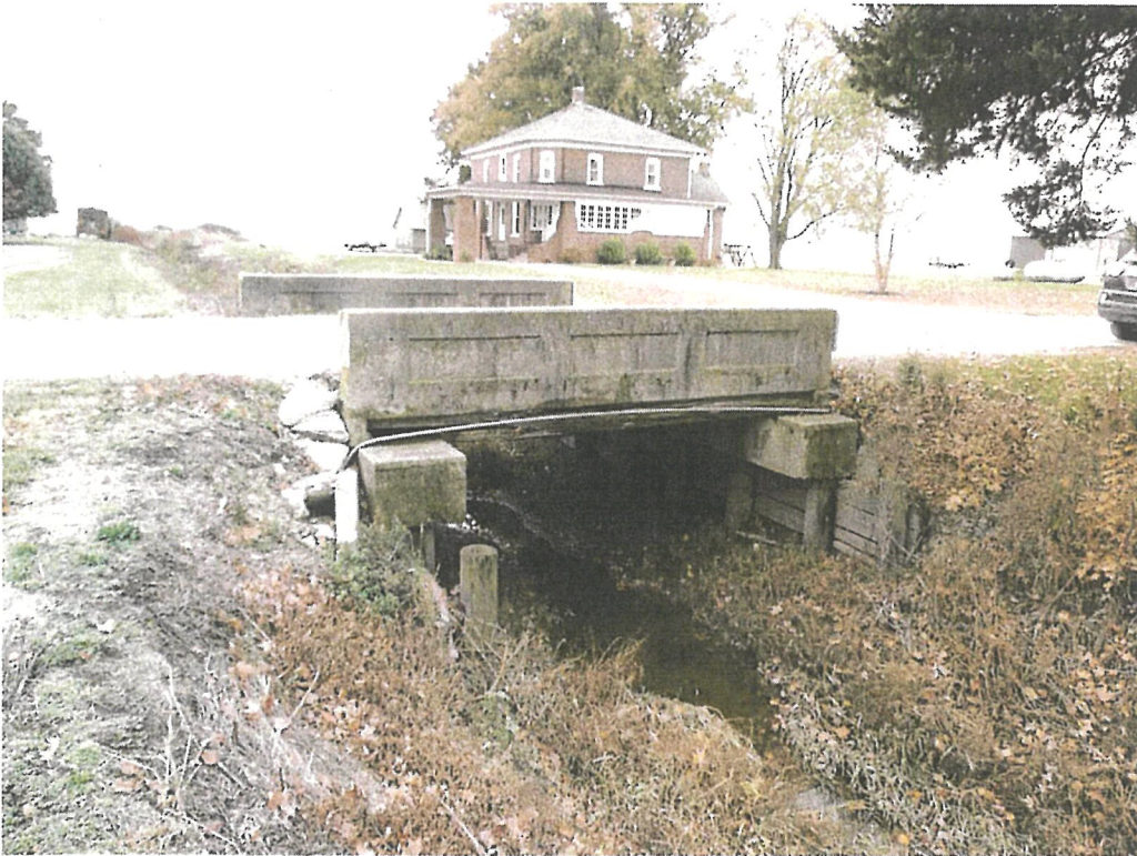
Prairie 2725E 600N Replace with Rebuild Illinois Funds – 13.83 feet x 6.58 feet
